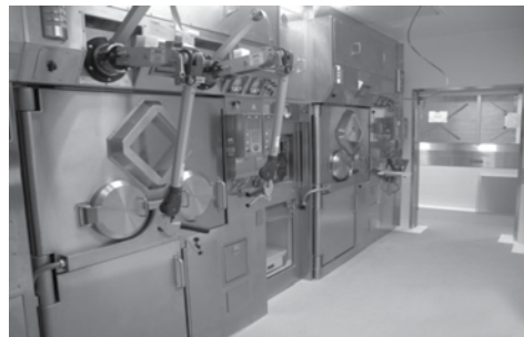
The new Lu-177 production suite hot cells
